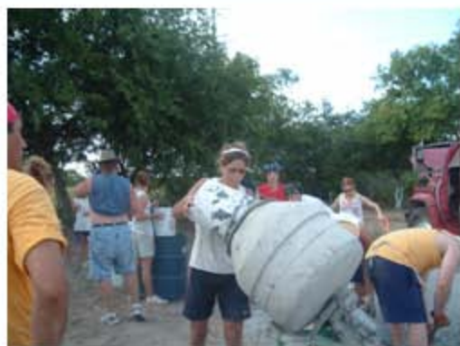
Smyser Team mixing cement for footing for new church building in Matamoros
