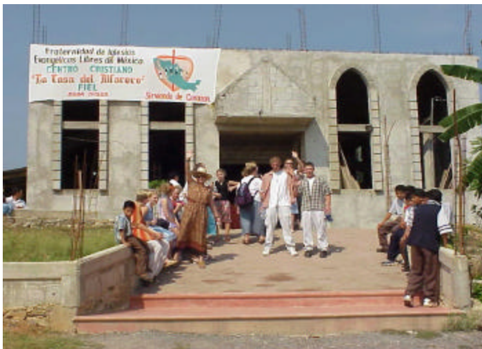
Smyser Christian Church members celebrate the cement floor being poured in El Alfarero Church in San Felipe, Hidalgo, Mexico.
